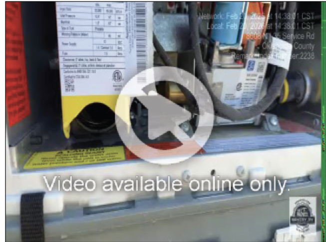
O-ring Seated No Leak
