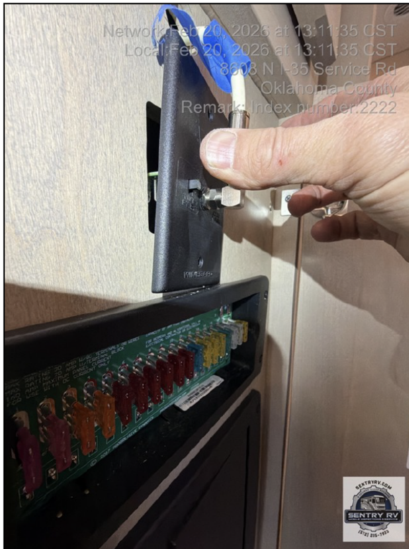
Coax Wall Plate Not Mounted
