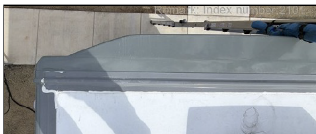
Rear Cap Joint Curbside
