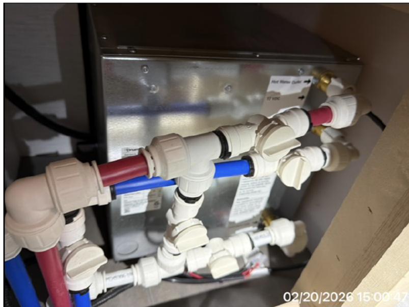
Water Heater By-Pass System
