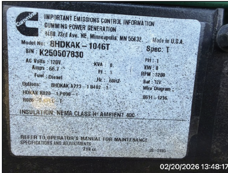
Generator Data Tag
