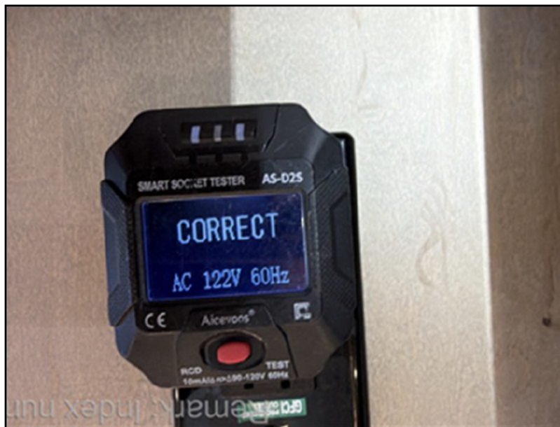
Inverter Power Test
