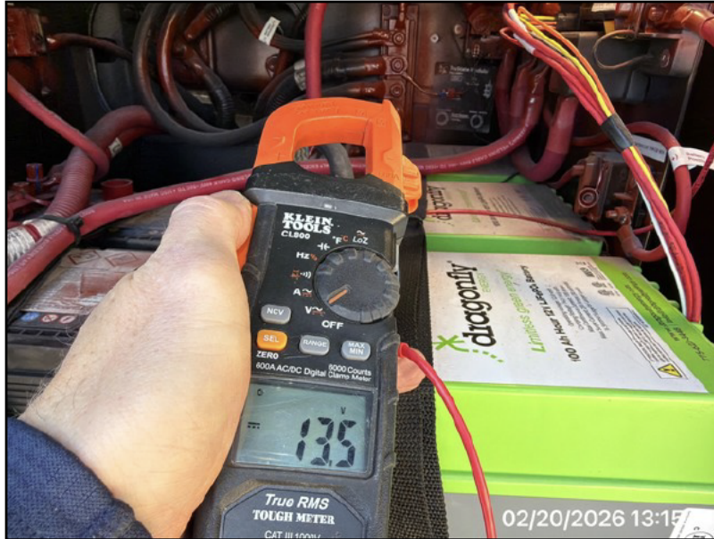
Battery Voltage Shore Power ON
