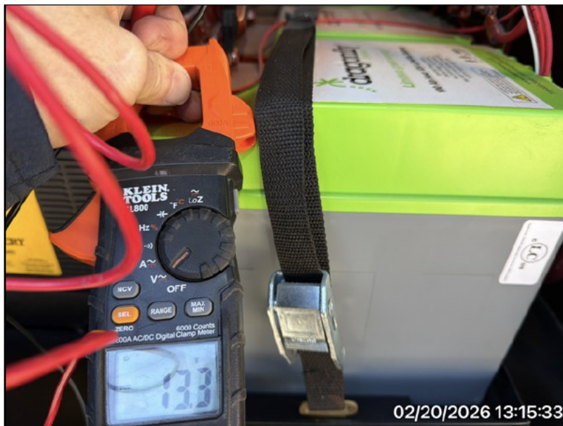
Battery Voltage Shore Power Off
