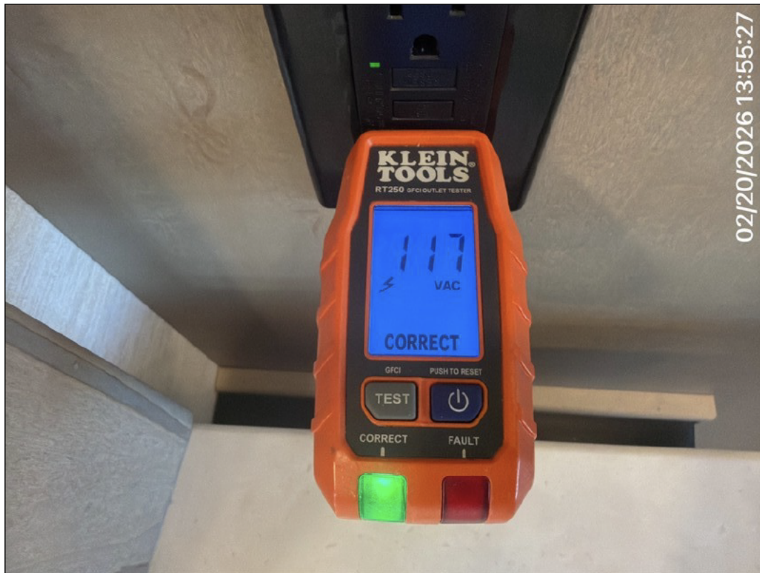
Gen Voltage Under Load
